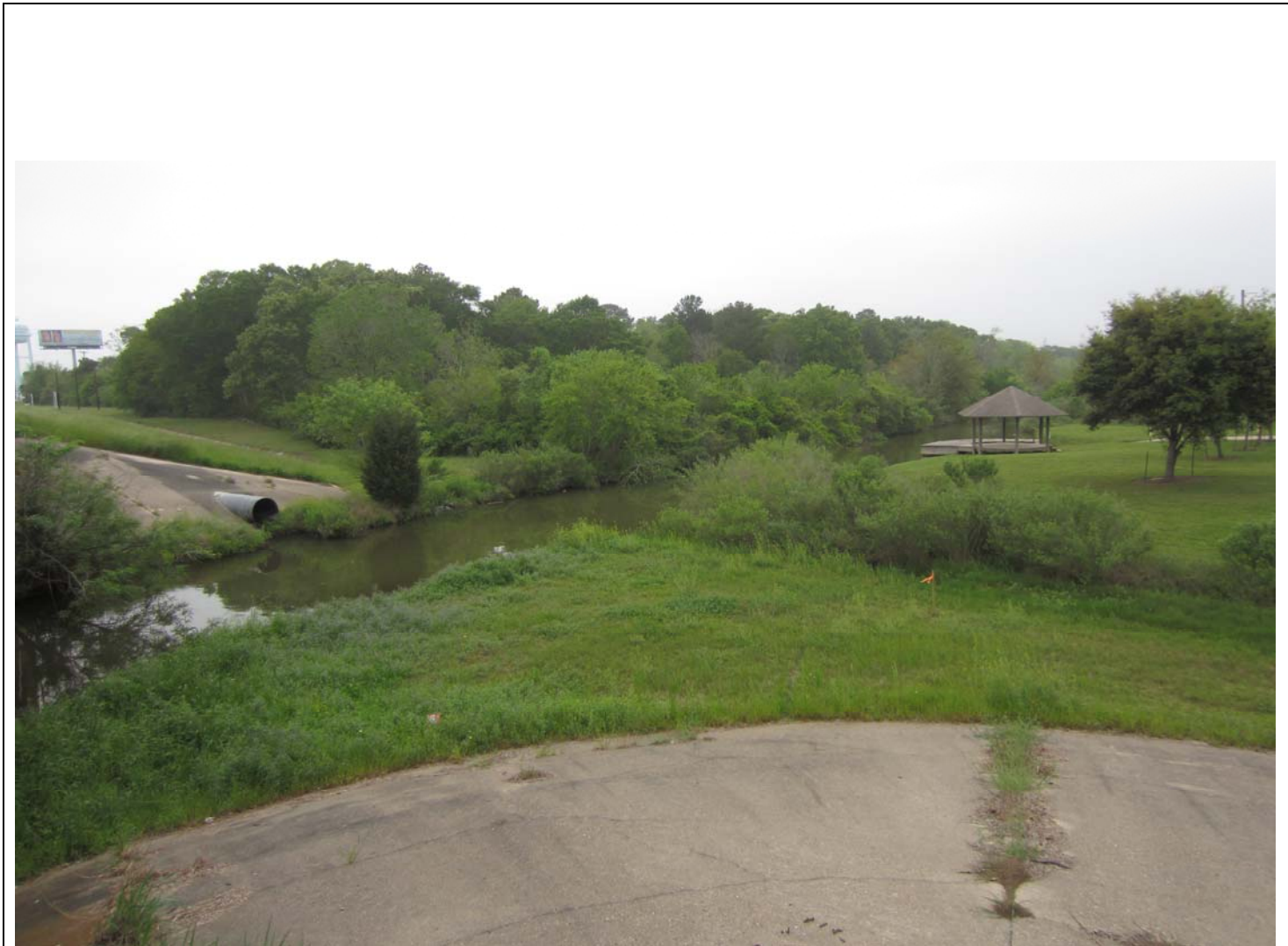
Robinson Bayou Downstream of the Proposed Bikeway/Pedestrian Bridge – Looking Northwest from the East Overbank.
