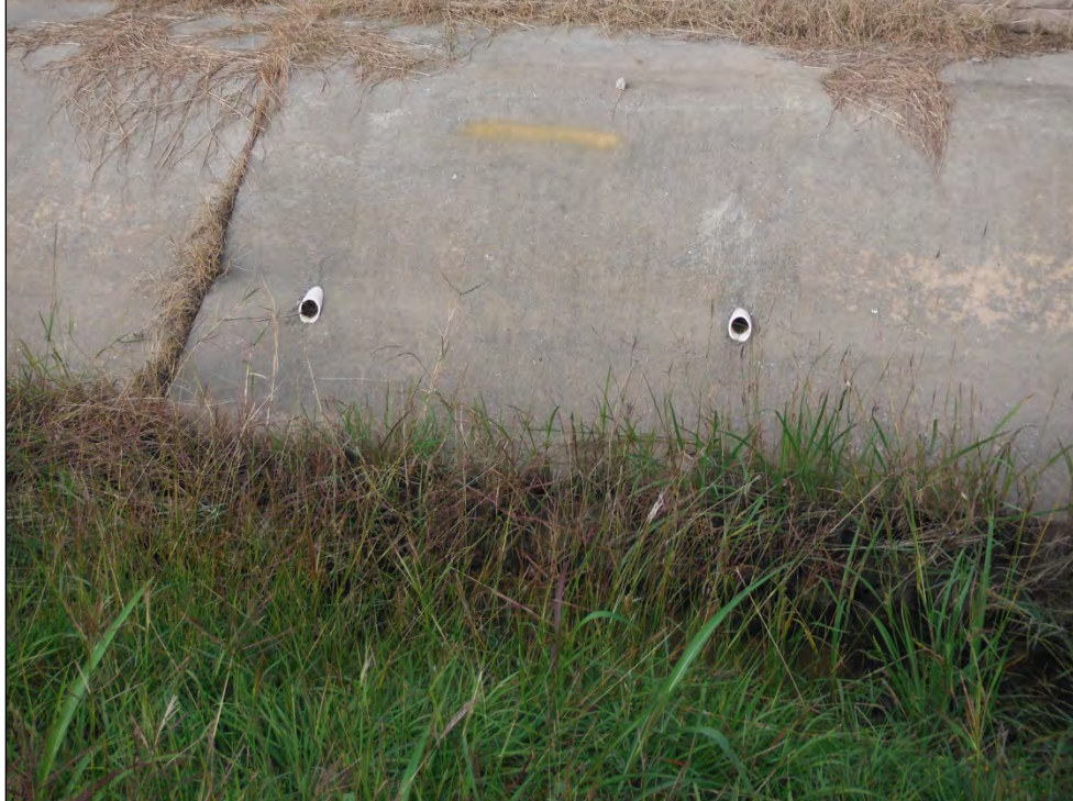
Facing west, this is a view of the PVC pipes that appear to drain runoff from the East Purification Plant into the roadside ditch.
