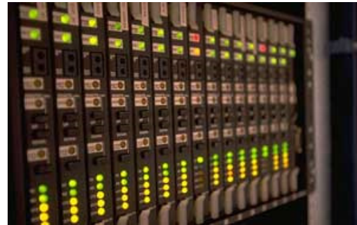
Figure 6-1 Telecommunication Rack—Lights Indicate Status
