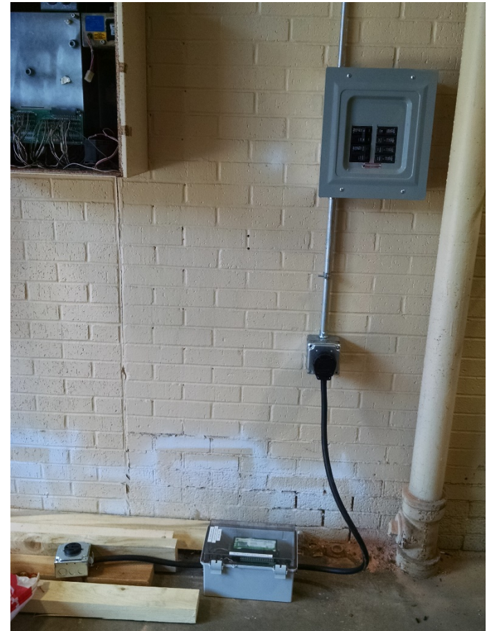
Meter connected between outlet and charge cord at TSU garage bay
