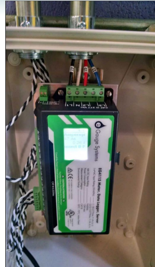
^Photo of an INL owned eGauge installed at another automated shuttle charging circuit
