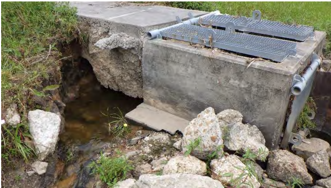
Figure 3: Bank collapse at water diversion
