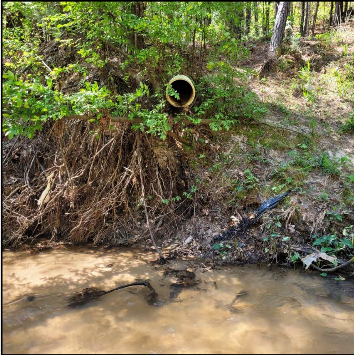
Figure 7: Referral site 23_WOC_FS_11. Pipe dripping into AU.
