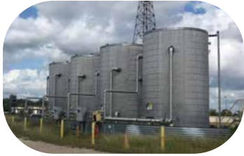
Rainwater Collection Existing Tanks
