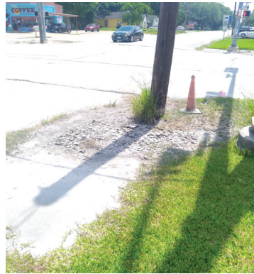
Existing Cracked Sidewalk and Poor ADA Facilities
