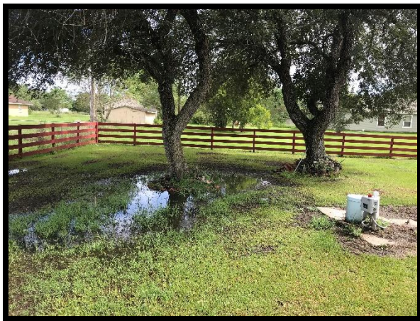
Figure 4. Failing onsite sewage facility
