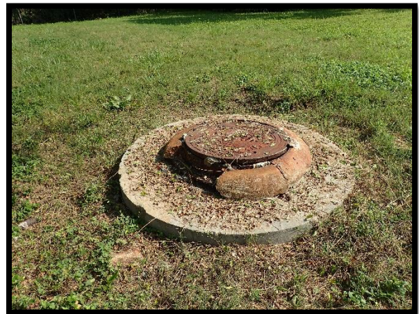
Figure 9. Aging infrastructure with evidence of sewage overflow
