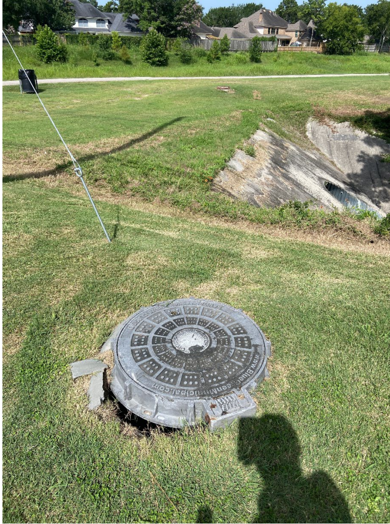
Figure 12. Broken Manhole Cover at Faulkey Gully (1009C)
