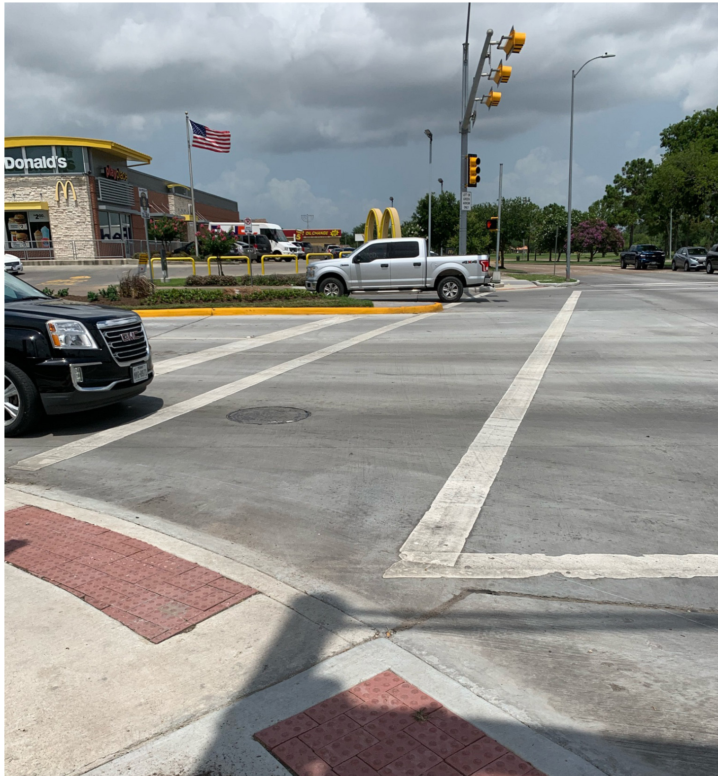
The existing intersection at Hillcroft Avenue and S. Braeswood Boulevard is auto-oriented and should be redesigned to be safer for all modes of transportation.
