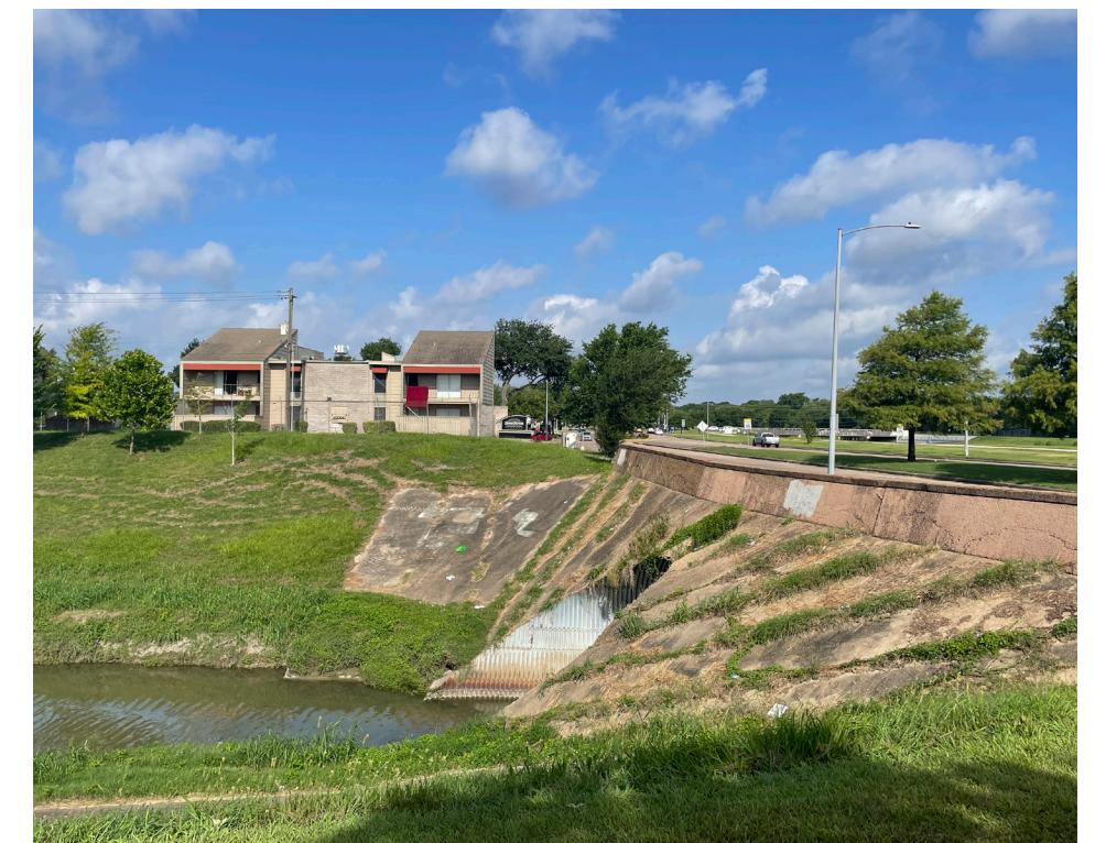
Storm sewer line as seen in the study area.
