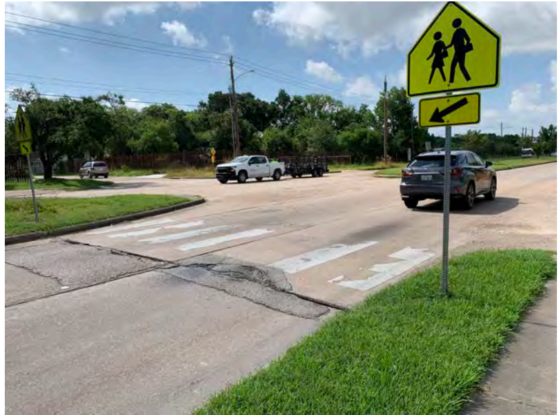
Figure 36: Marked school crossing on S. Gessner Road with no ADA ramps
