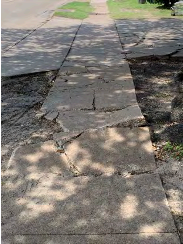
Figure 6: Broken sidewalk along South Gessner Road
