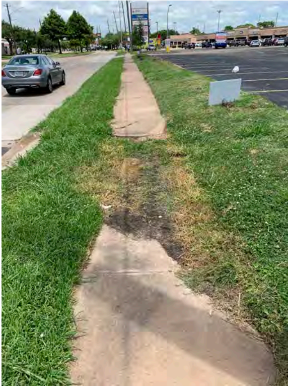
Figure 37: Broken/missing sidewalk along West Bellfort Avenue was given a poor rating
