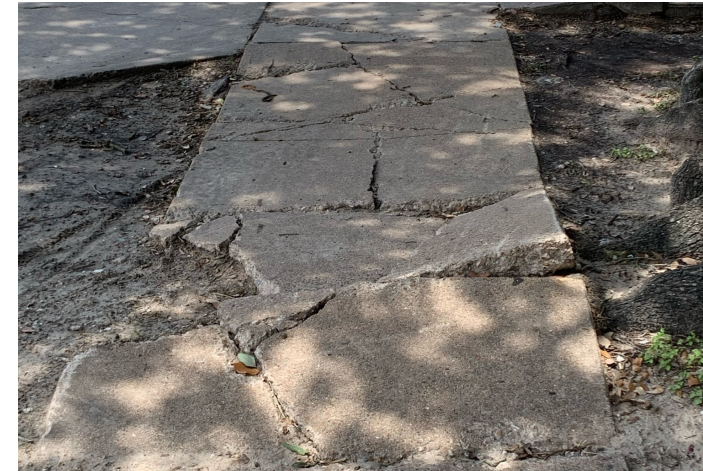
Lighting along and the sidewalks are missing. Some sidewalks need repair.
