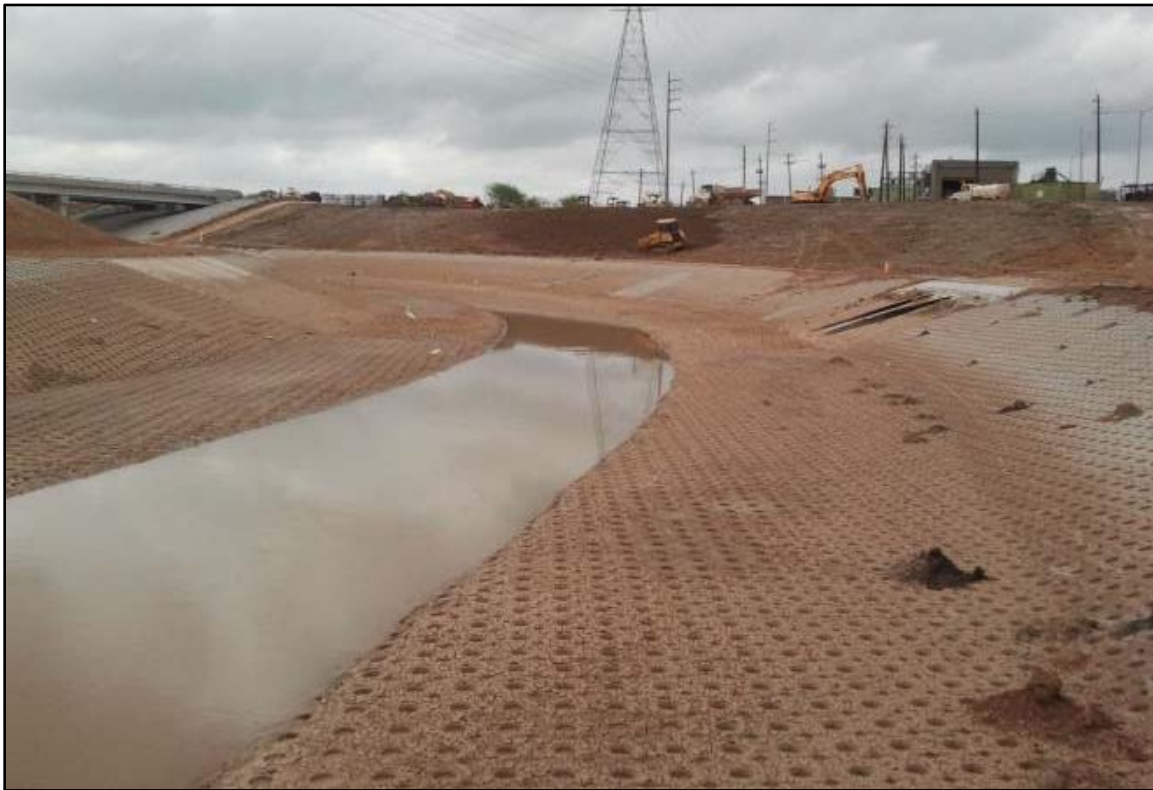
Figure 17. Photo of construction work under the Federal Flood Damage Reduction Project on Sims Bayou at W Orem Dr. Photo courtesy of U.S. Army Corps of Engineers - Galveston District U.S.
