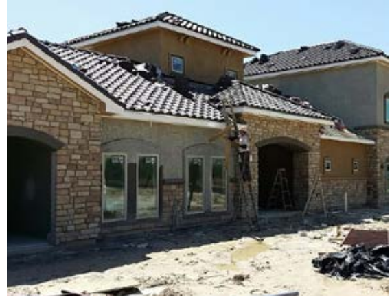
Renovation of the Gulf Coast Arms apartments in 2014 using Low Income Housing Tax Credit Funds. (Image: The Brownstone Group)
