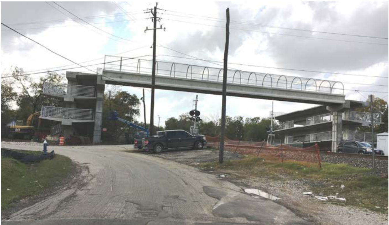
The Bringham Street bridge is under construction with both accessible ramps and safety cages.
