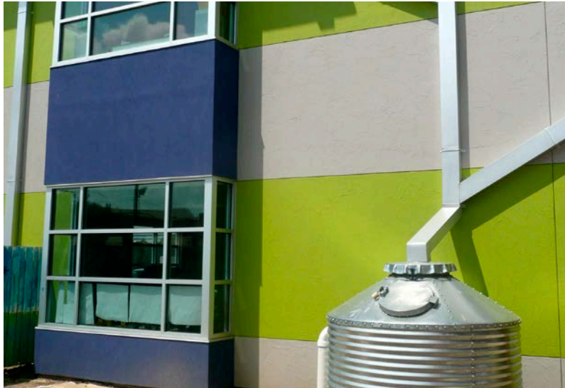
BAKER RIPLEY rainwater harvesting
