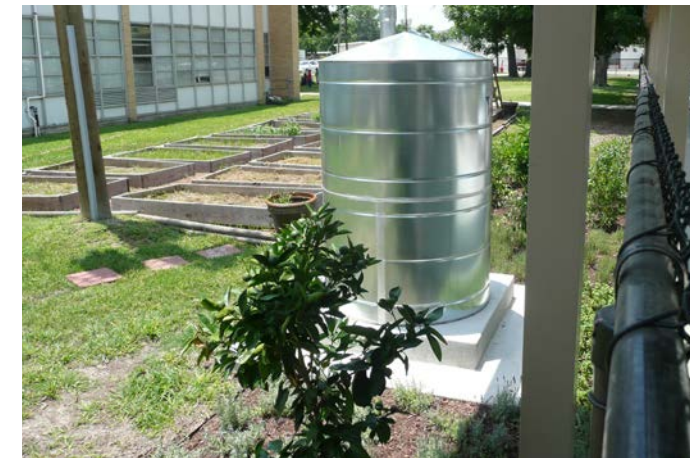
ROSS ELEMENTARY rainwater harvesting
