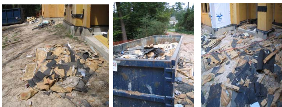
Figures 22-24. Asphalt shingles from Haul Three
