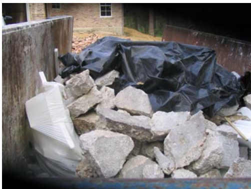
Figure 38. The unacceptable flatwork
