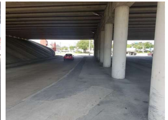
Both sides — 2.5' diam. columns, centered in 20' back of curb to back of curb, spaced at 16' C-C
