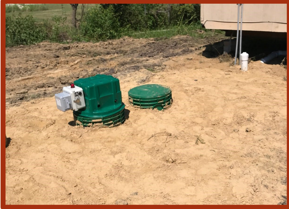
New aerobic OSSF
