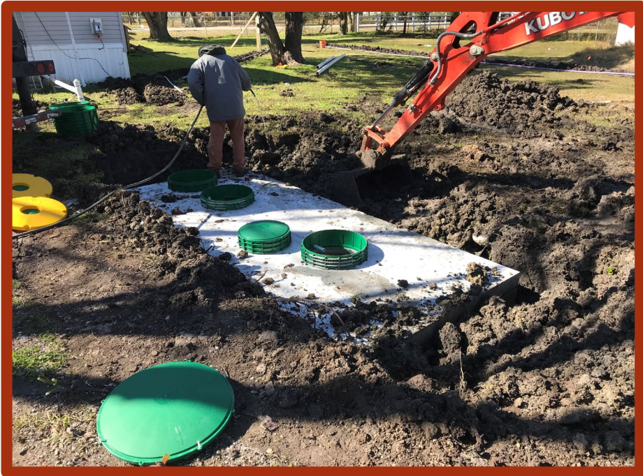
New aerobic OSSF
